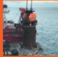
NOT LEAVING PILE DISCONNECTED RESTING IN GRIPPER OF TEMPLATE/JACKET SLEEVE
